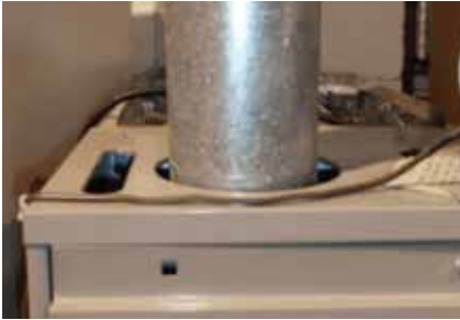
Low-efficiency furnaces vent through metal pipes
