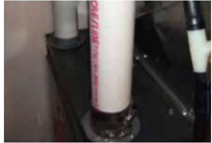
High-efficiency furnaces vent through plastic pipes
