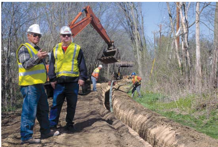
Crews installed a new gas line in the Mount Horeb area to meet energy needs in the expanding communities in western Dane County.
