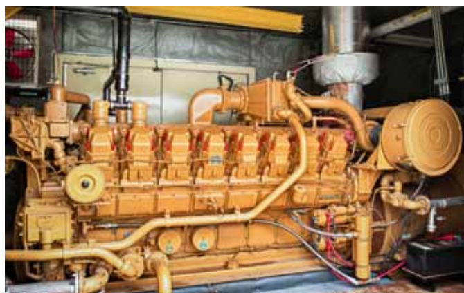
This is a 1,600-kilowatt generator located at the Rodefild Landfill on Madison's southeast side. It helps convert methane gas into electricity, which MGE buys and uses to power more than 4,500 homes.
