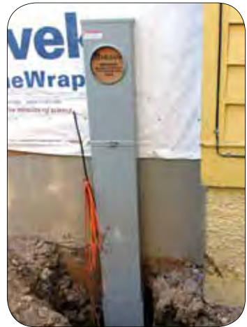
Meter socket installed with cable TV and telephone wires waiting final connections
