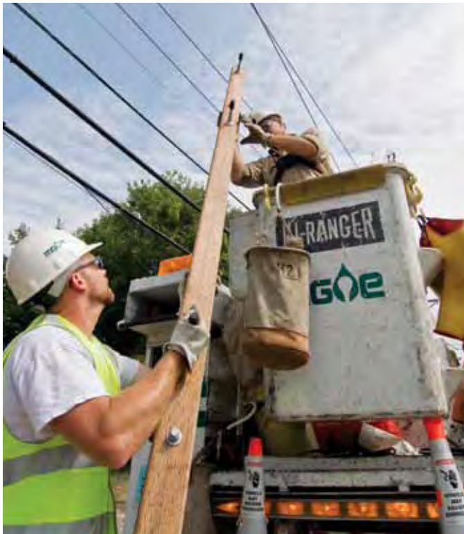
Regular maintenance is critical for a reliable electric system. Rob Priestley (left) and Bob Harper, MGE line technicians, replace a power pole.
